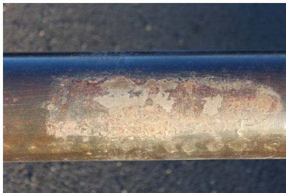
Pic # 3. Surface rust
